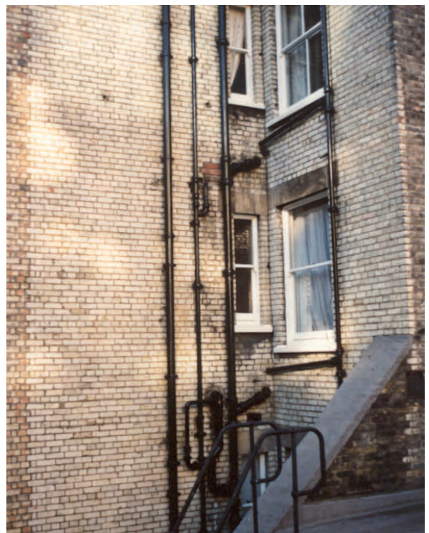
Figure 9: White walls require regular maintenance or their reflectance will deteriorate, as shown here
