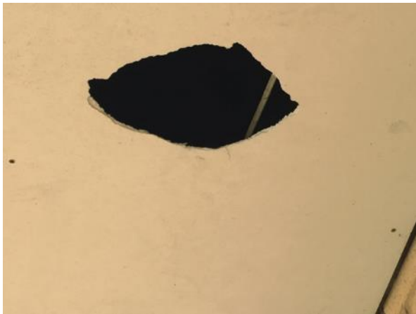
Plate 13 TN6: Substantial gaps in underside of roof allowing bird and bat access
