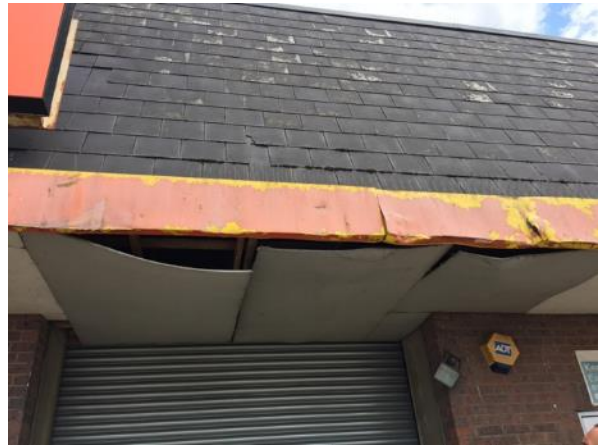
Plate 12 TN6: Substantial gaps in underside of roof allowing bird access
