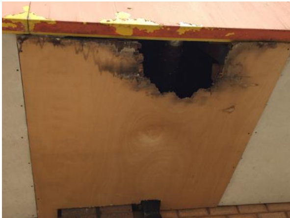
Plate 11 TN6 Cavity with visible bird droppings and feathers inside
