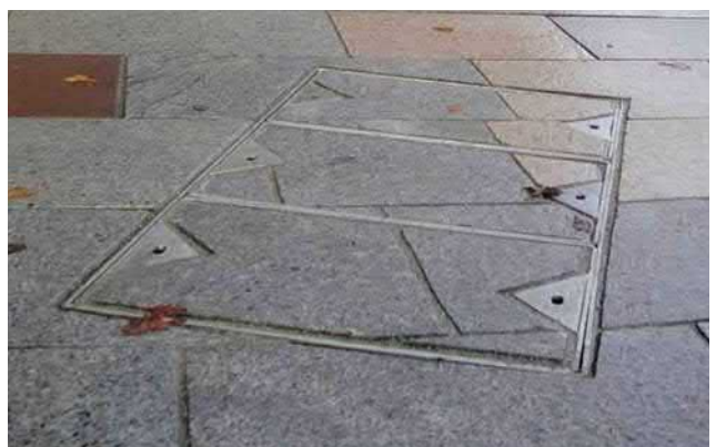
✗ Non-recessed manhole covers not aligned with paving pattern
