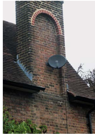
▲ A poorly sited dish on a prominent chimney.
