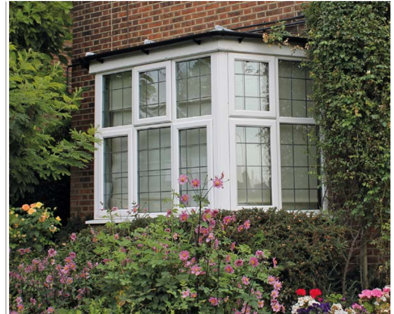
▲ A UPVC bay window. This looks nothing like the steel and timber bay it replaces and detracts significantly from the house.
