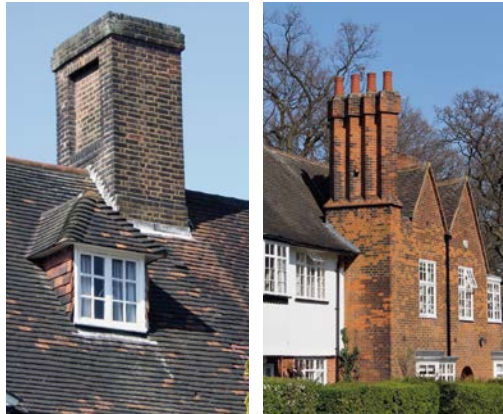
▲ Examples of prominent chimneys. Their design reflects the importance of the open fire in heating early Suburb houses.
