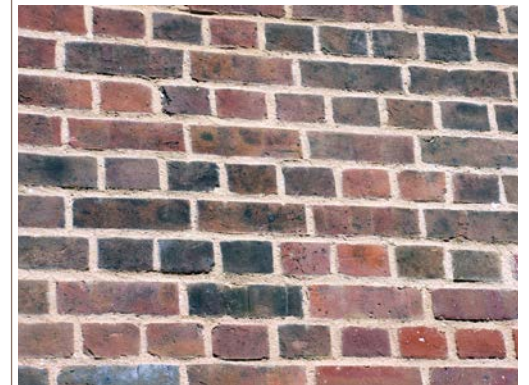
► Good pointing. Soft lime mortar in a pleasant buff colour is finished slightly recessed behind the face of the bricks and brushed to expose the texture.
