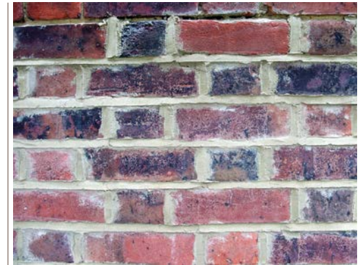
► Very bad pointing in grey cement mortar. The mortar is smeared over the face of the bricks and the work is untidy.
