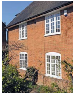
▲ A good timber double glazed replacement window next to an original window.
