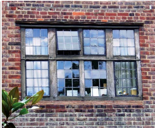
▶ Examples of leaded windows showing the differing reflections. This lively appearance, which adds so much to the character of these houses, cannot be replicated in double glazed windows.
