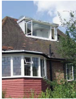
▲ This dormer is too large, poorly designed and too high in the roof.
