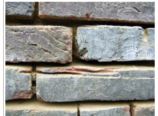
► Bad cutting-out with a mechanical grinder. The bricks have been badly damaged and the joints widened.
