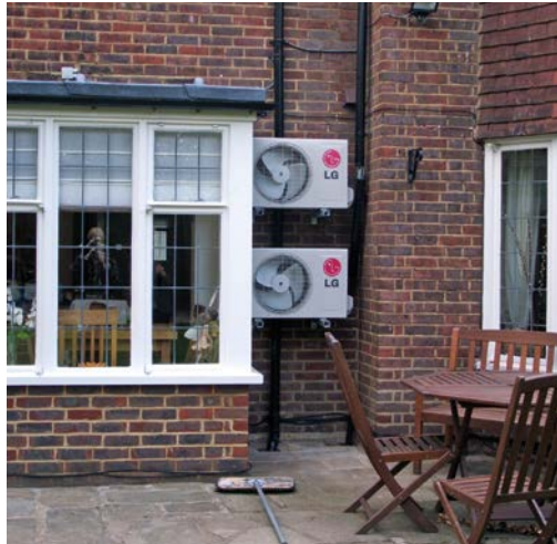
▲ Poorly placed air conditioning units can spoil an attractive elevation
