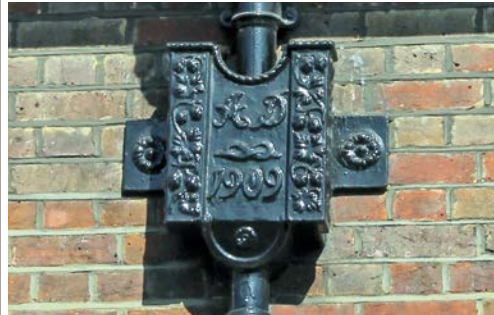
▼ Decorative hopper heads are evidence of the care exercised by the Suburb's architects. They must be retained.
