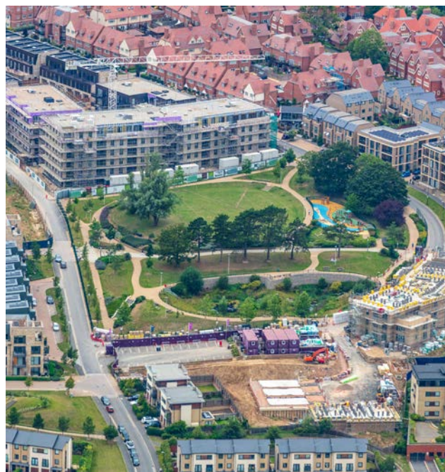
» Mill Hill East Phase 5 (Joseph Homes) construction foreground & Phase 4a and 4c (Taylor Wimpey) under construction
