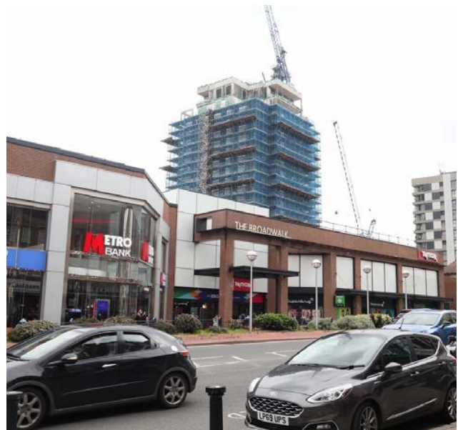
» Edgware High Street view of Broadwalk centre, refurbished block and new block under construction
